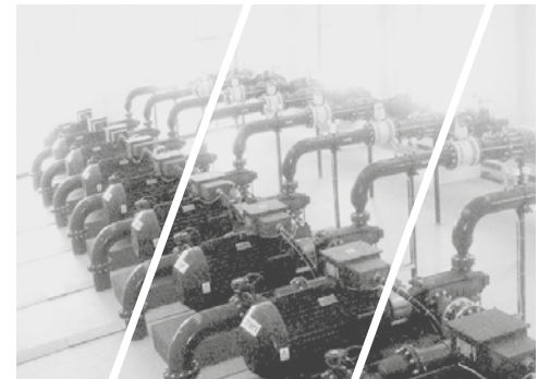
Boosting and Distribution of surface water
